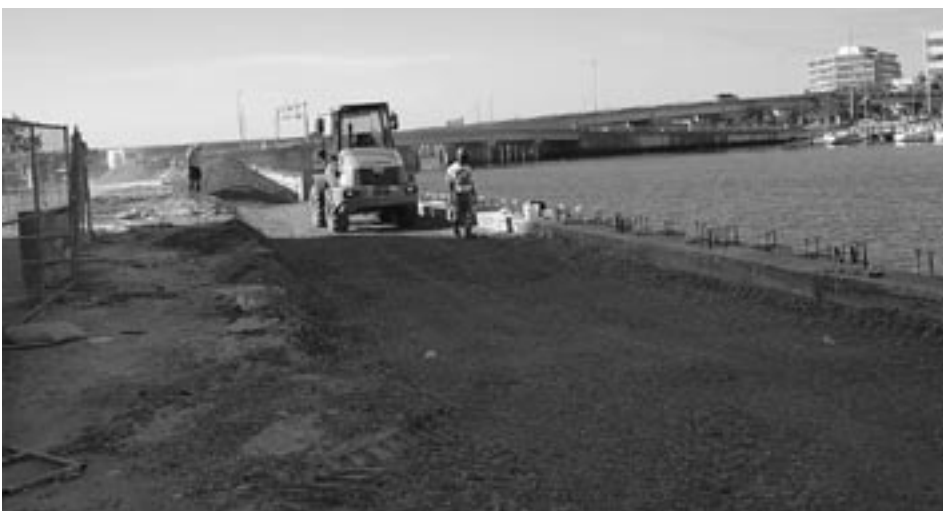
Workers prepare a temporary road to route vehicles around the construction zone. The road, which recently opened to traffic, will eventually be replaced by a permanent road around the new building.
