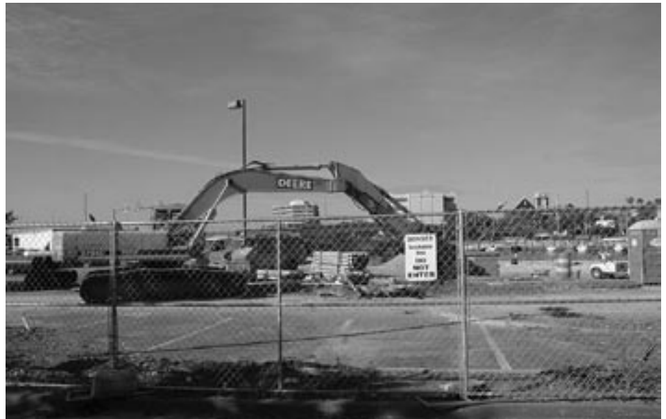
The northwest side of Tampa General's campus is now a construction zone as workers prepare the site for groundbreaking.
