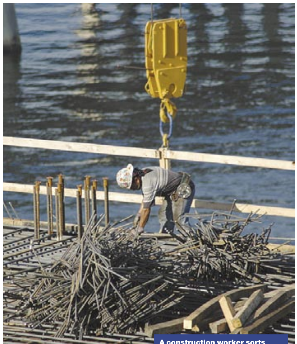
A construction worker sorts metal rods used to reinforce the building's concrete floors.
