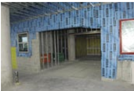
The entrance to the Emergency and Trauma Center from the ramp. Automatic doors will be installed later. Visitors and ambulances can bring patients right to the door.
