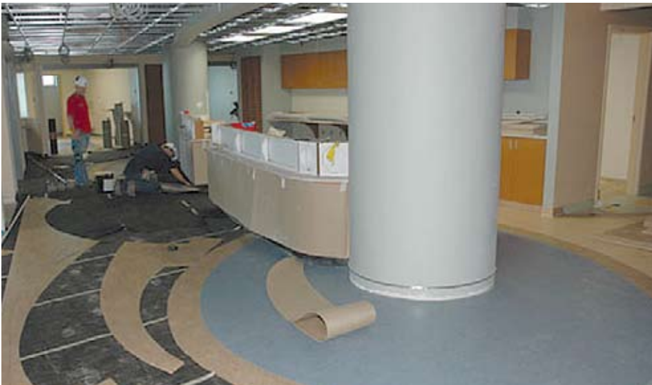
Workers lay the flooring around a nursing station for the new Neurosciences Intensive Care Unit on the fifth floor.
