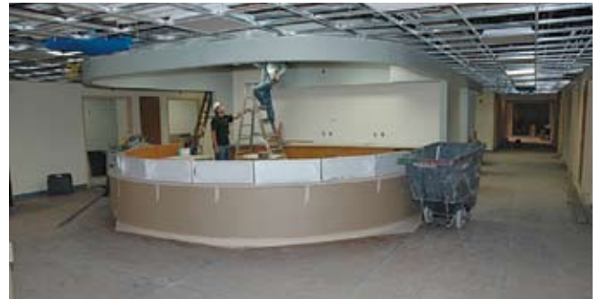
A nursing station on the second floor Emergency and Trauma Center. The center's 72 patient rooms will be divided among 10 pods, each with its own nursing station.
