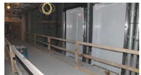
These newly installed staff elevators are located on the new building's north side and will be accessible from within the West Pavilion. Visitors will take elevators on the building's south side.
