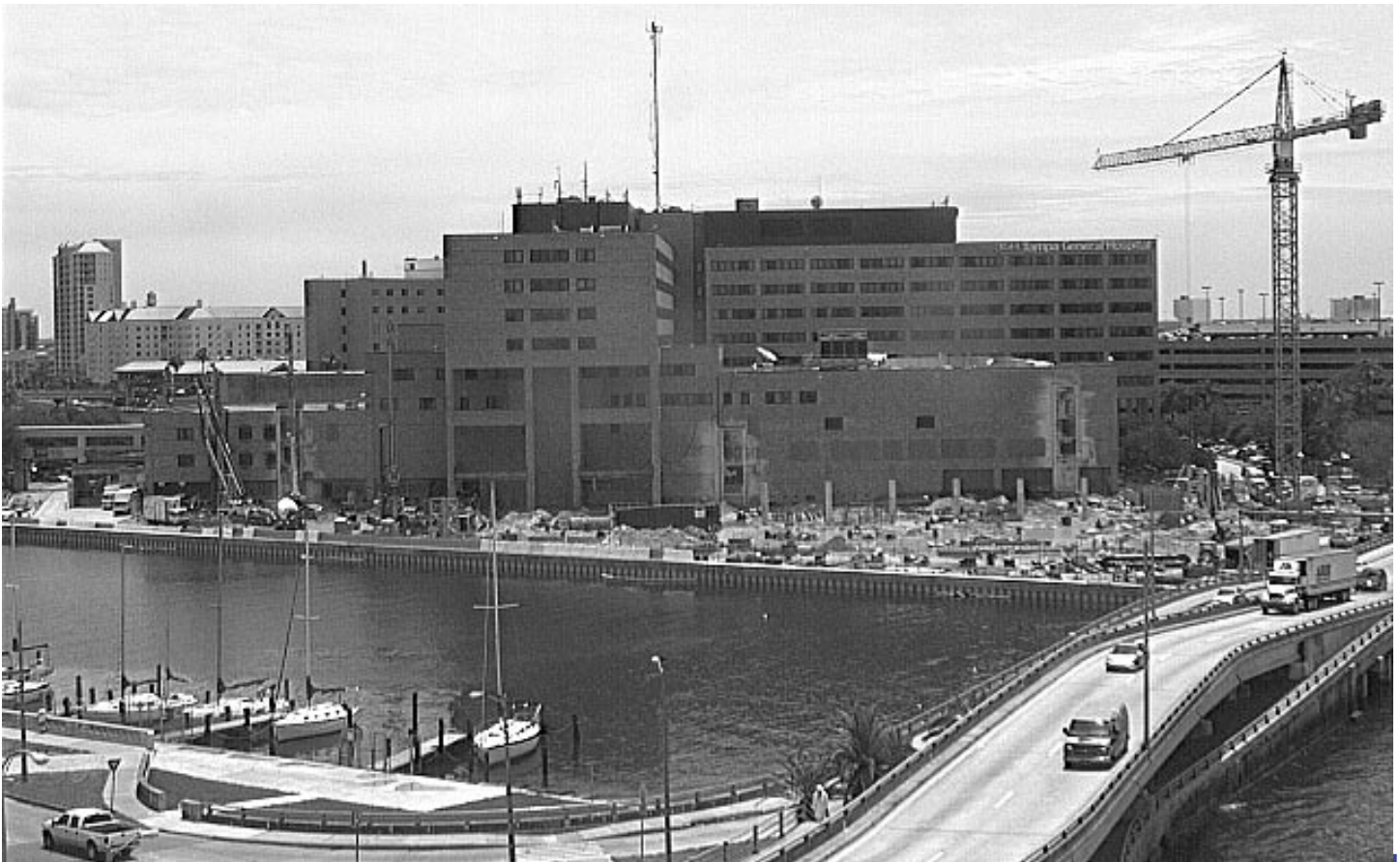
The expansion project is well underway at Tampa General, with workers beginning to shape its structural frame.
